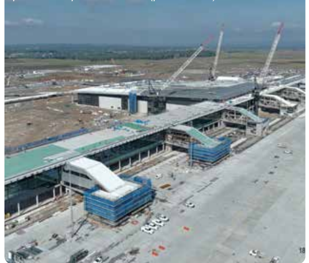
Western Sydney International Airport is planned to open in late 2026 (photo: WSI).
